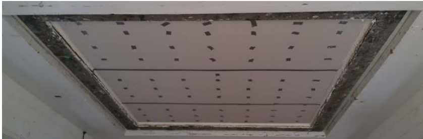
Photo 2: View of Receive Chamber, gypsum panel ceiling observed
