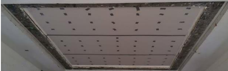
Photo 2: View of Receive Chamber, gypsum panel ceiling observed
