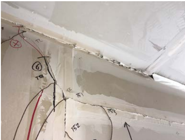
Photo 1 shows the results of the traditional method at the non-fire side where the paper tape cracks and pulls apart which in return allows smoke to pass through the head-of-wall joint.
