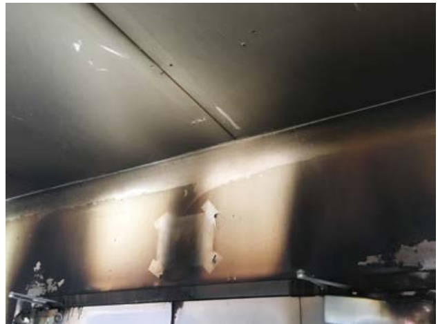
Photo 2 shows the HOTROD Compressible Firestopping on the non-fire side. Although the double metal door failed and allowed fire and smoke to pass through the door, fire or smoke was unable to pass through the head of wall joint as indicated in the clean, off white seal line between the ceiling and the wall.
